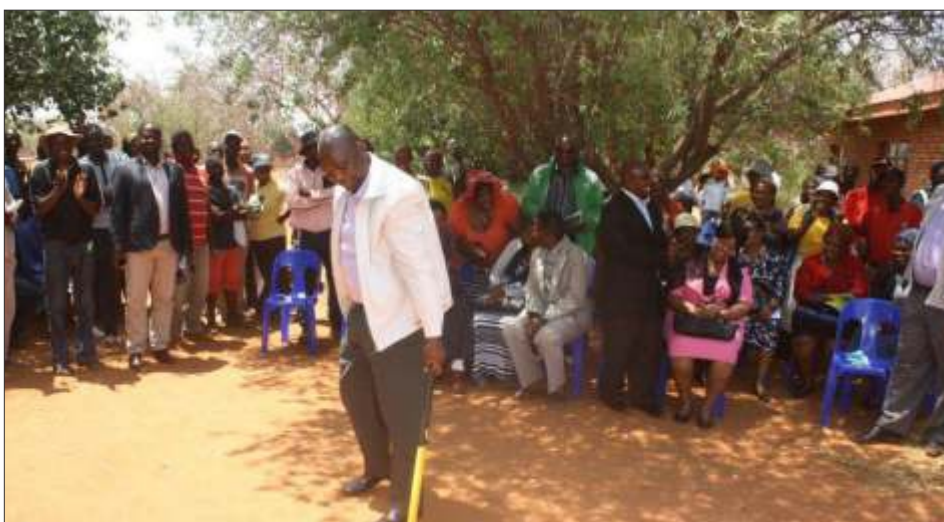
Mayor Selamolela breaks ground marking the commencement of the construction of Taaibosch Waste Transfer Station.
